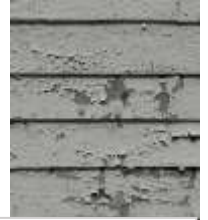
Deteriorating paint before the restoration
